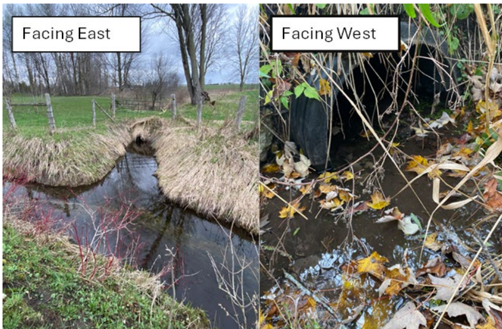
Figure 3: Existing Culvert to be Removed on Lot 33 Conc. 8, Howick, (Roll 0-042) Bradley & Lindsey Hall property
