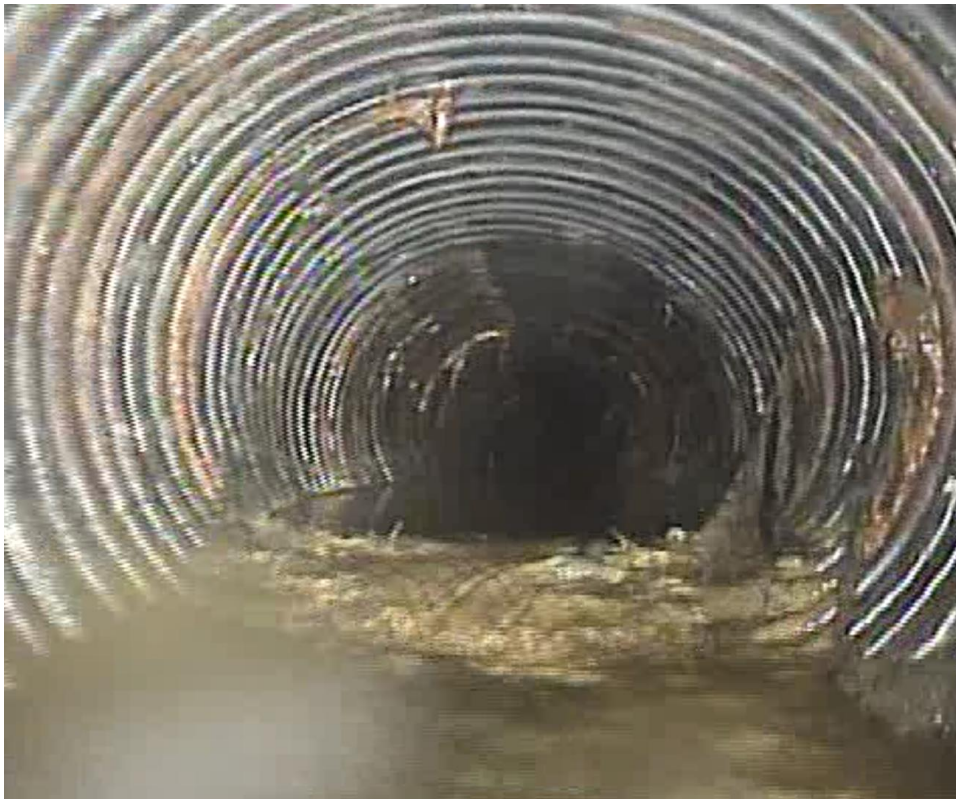
Figure 6 – Root growth in Main Drain tile through woodlot on Lot 7, Concession 8
