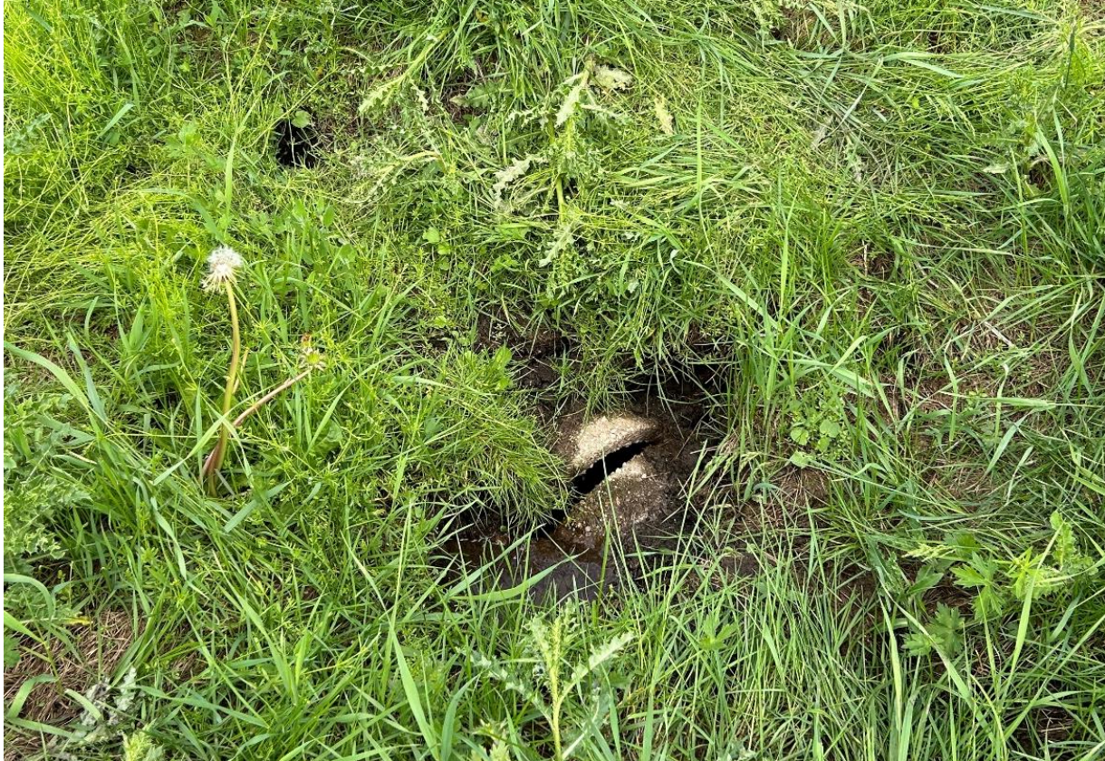
Figure 1 – Exposed 14" dia. concrete municipal tile in the low-lying lands on Lot 7, Concession 8
