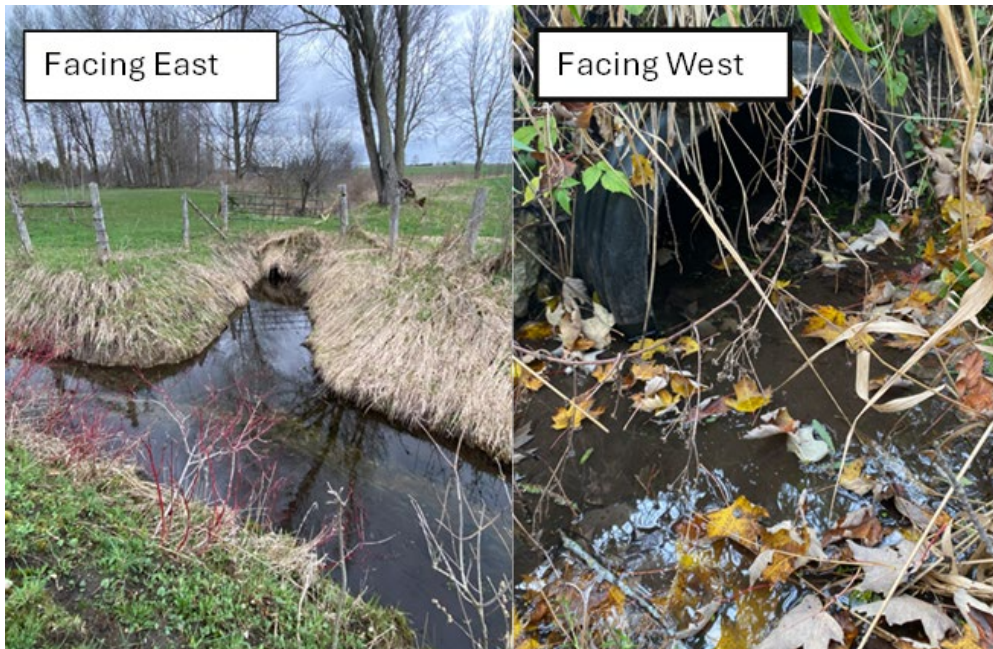
Figure 3: Existing Culvert to be Removed on Lot 33 Conc. 8, Howick, (Roll 0-042) Bradley & Lindsey Hall property
